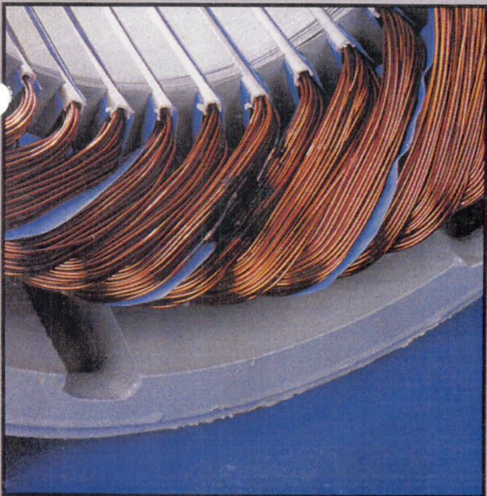
3 Winding Shorted Phase-To-Phase
