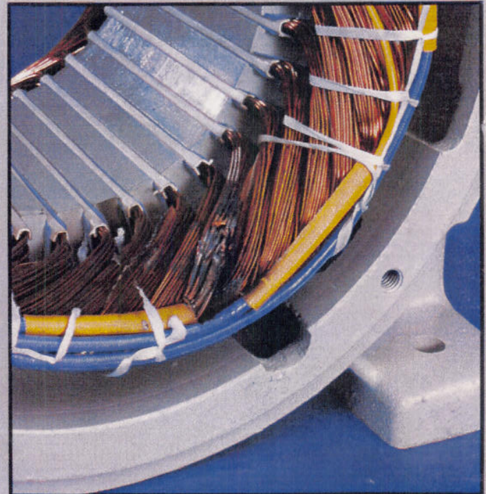
12 Winding Damaged by Voltage Surge
